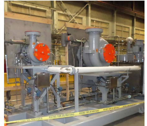
Rotoflow cryogenic expander installed in a small-scale LNG plant.
