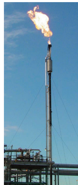
Flare Testing Upper Steam Flares
